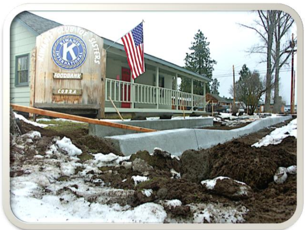
Oak St. And E. Main Ave. undergo improvements to the curbs and bump outs. Parking in front of our Kiwanis House will become “back in” slots to enhance traffic safety
